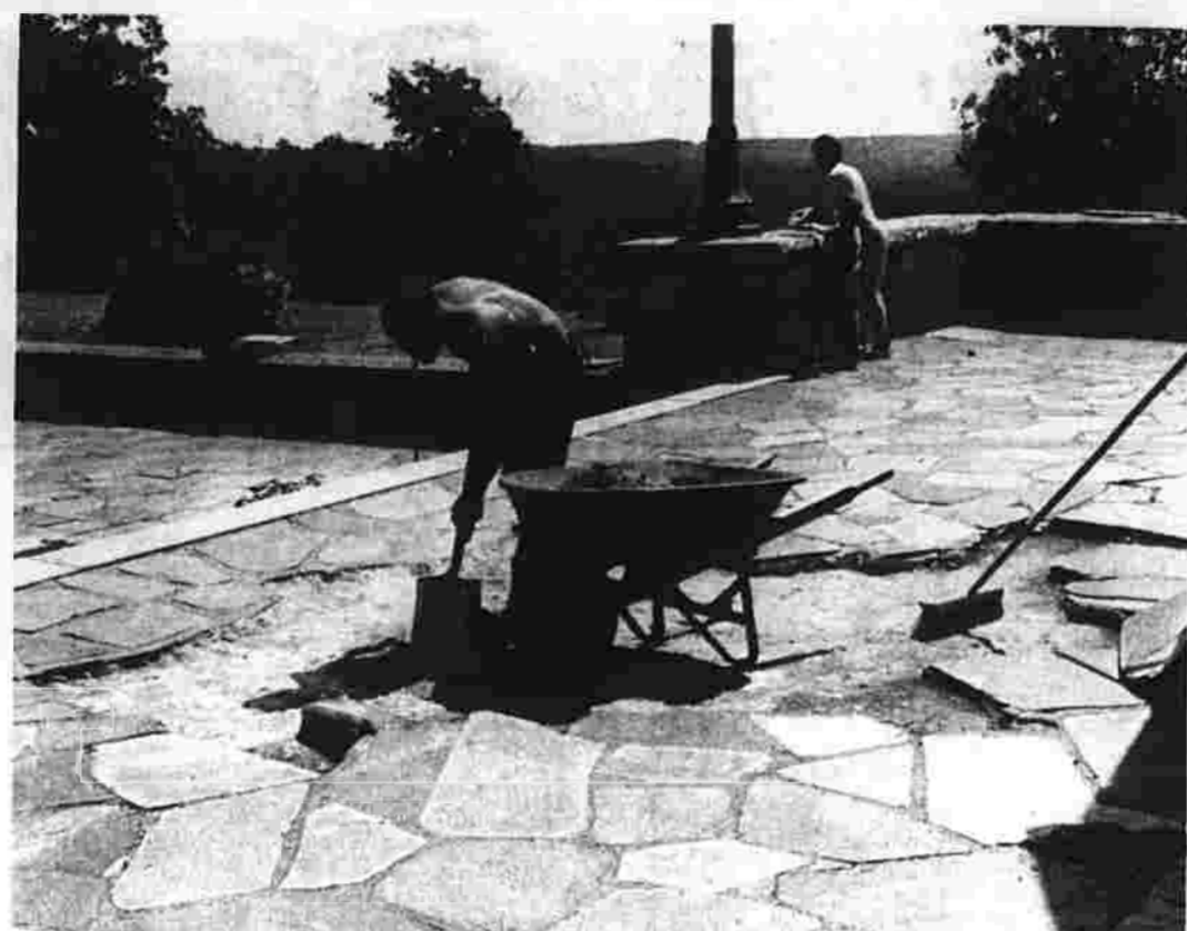
A cement worker of the Volpe Co. cleans out an area of flagstone in front of the Fox Hill Tower at Henry Park, Rockville, while in the background a man and a boy enjoy the view. Repairing the walkway is part of a program in preparation for again opening the tower for public use. (Herald photo by Richmond)
