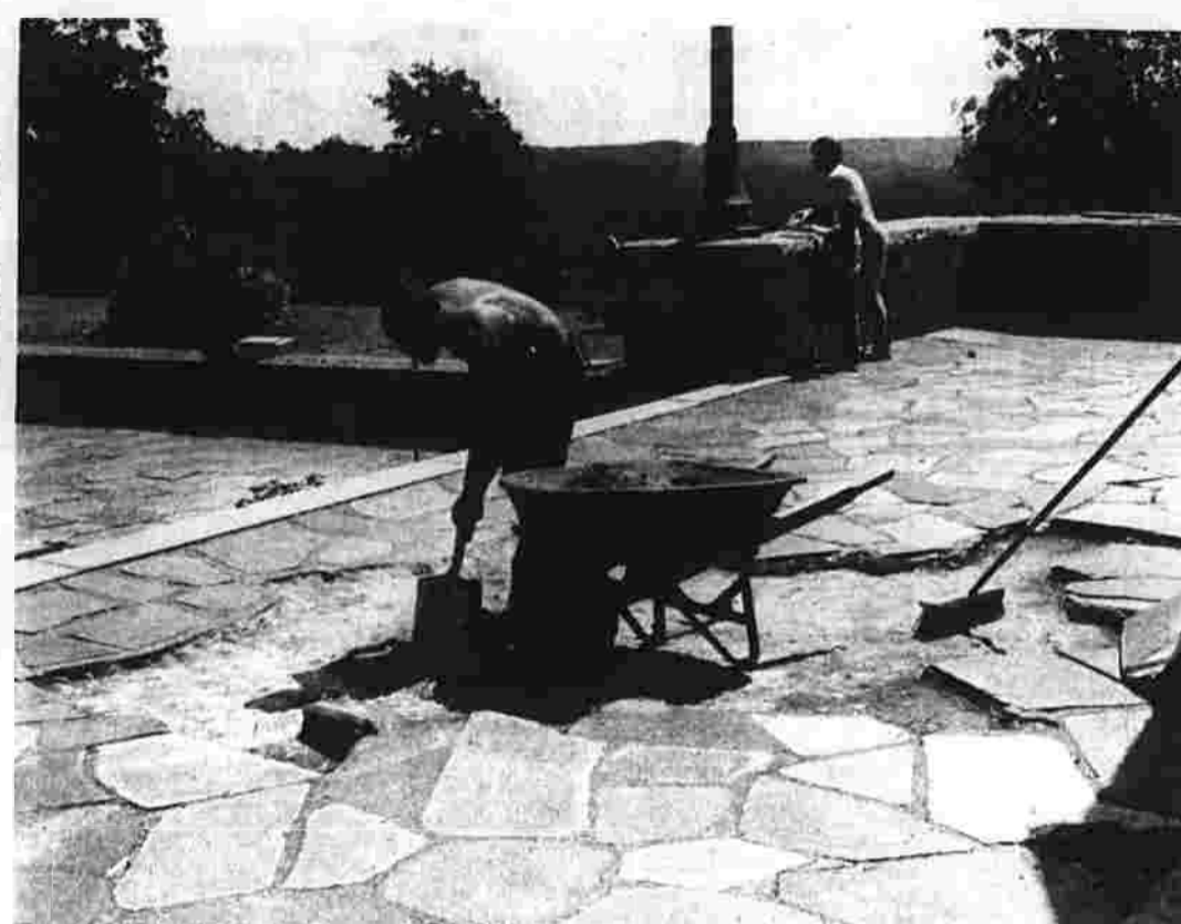
A cement worker of the Volpe Co. cleans out an area of flagstone in front of the Fox Hill Tower at Henry Park, Rockville, while in the background a man and a boy enjoy the view. Repairing the walkway is part of a program in preparation for again opening the tower for public use. (Herald photo by Richmond)
